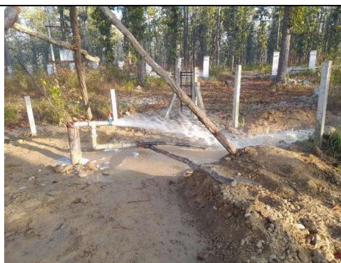
Figure 6 Lift drinking water- ward no 10
